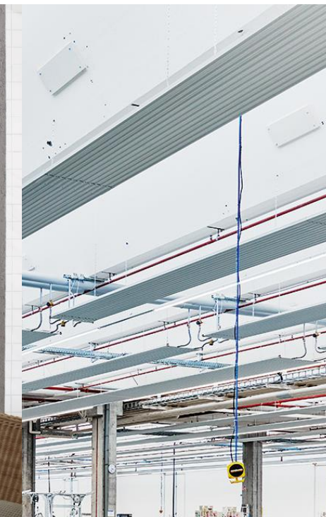
Heating & cooling panels
